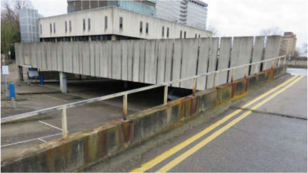
Southend Central Library car park. The rotting concrete wall is the site for Acarospora moenium . Photo © John Skinner
