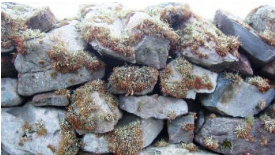
Photo 1. Storm-damaged Ramalina siliquosa , west-facing wall, Fair Isle, 8 th February 2017.
